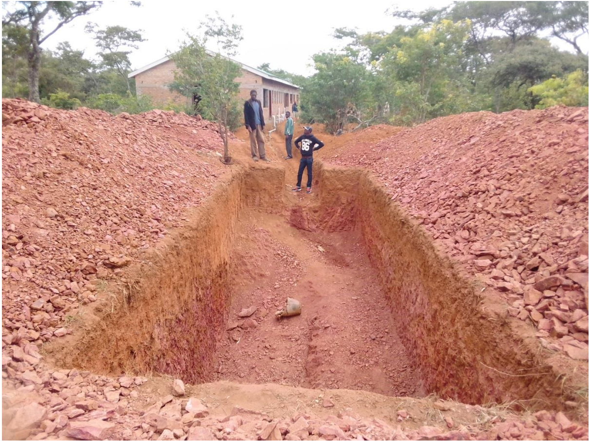
The Septic tank measuring 9m(L),3m (D) and 3 (W) still being dug. A soak way tank will be dug soon after the completion of the septic tank. The second hole will be measuring 3m (D) x 3m (L) x 2m (W).
